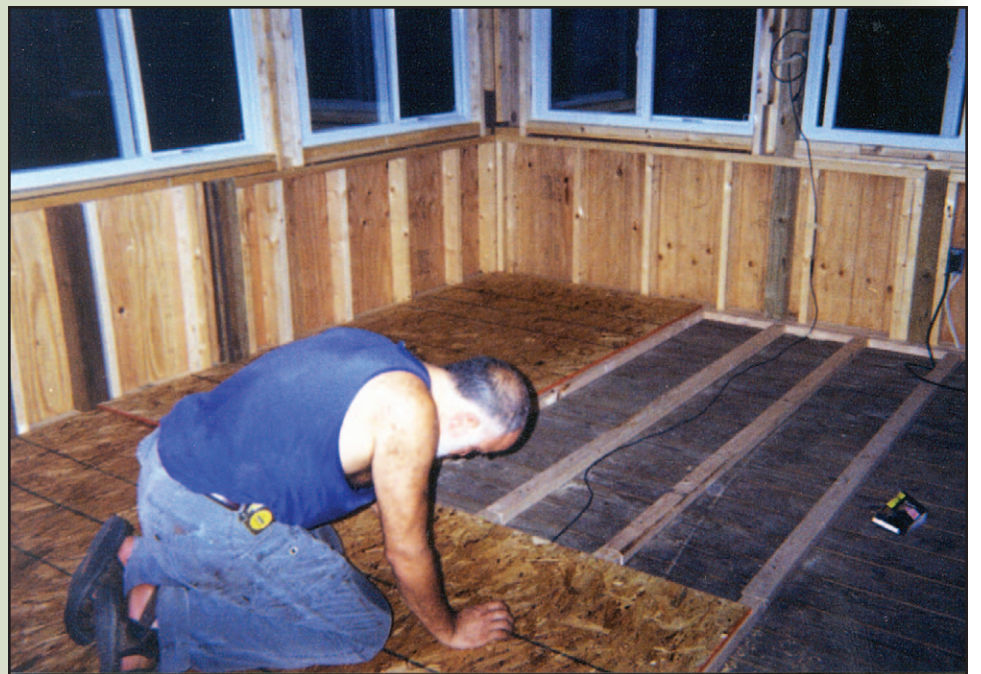
Laying a sub-floor over the existing porch floor required accurate measuring and cutting.
