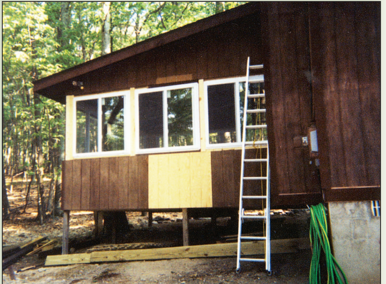
TRR photos by Marcia Nehemiah The unpainted siding shows where the door of the porch used to be. Standard-sized windows have been installed and framed.
